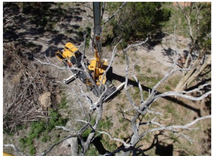
Photo 3: View from the man-box. Not a job for those afraid of heights
